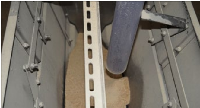
Feed comes directly out of the drop-down pipe.
